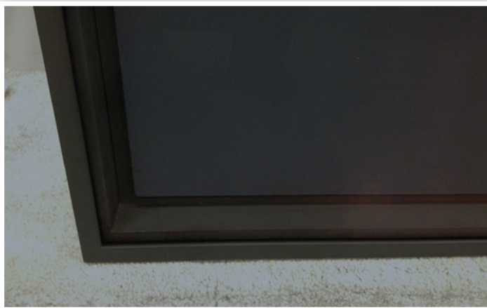
Bottom left corner detail of finished frame, showing original frame within new welded aluminum housing.
