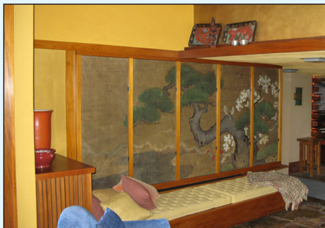
Photo of completed installation. Photo courtesy Ryan Hewson, Frank Lloyd Wright Foundation.
